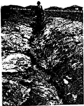
A Undermining of a spoon drain on the south bank of the creek near Sulby Place by surface runoff from the Westmeadows Bicycle Track. April 1977
