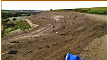
Looking east along the north wall, revegetation in progress. Retaining wall and the Creek to the left.
