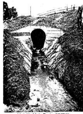
Melville Main Drain (MMBW)
